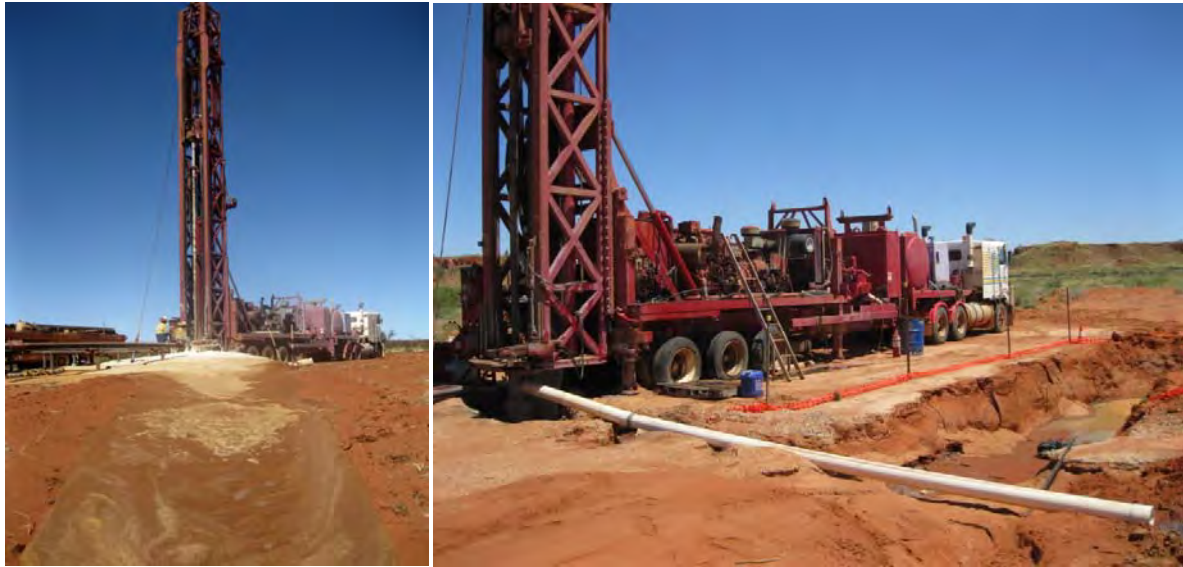
Figure 2-2: Heavy foam being ejected from CWB19 during drilling of the surface collar; discharge of cuttings and fluid flowing via a headworks apparatus
